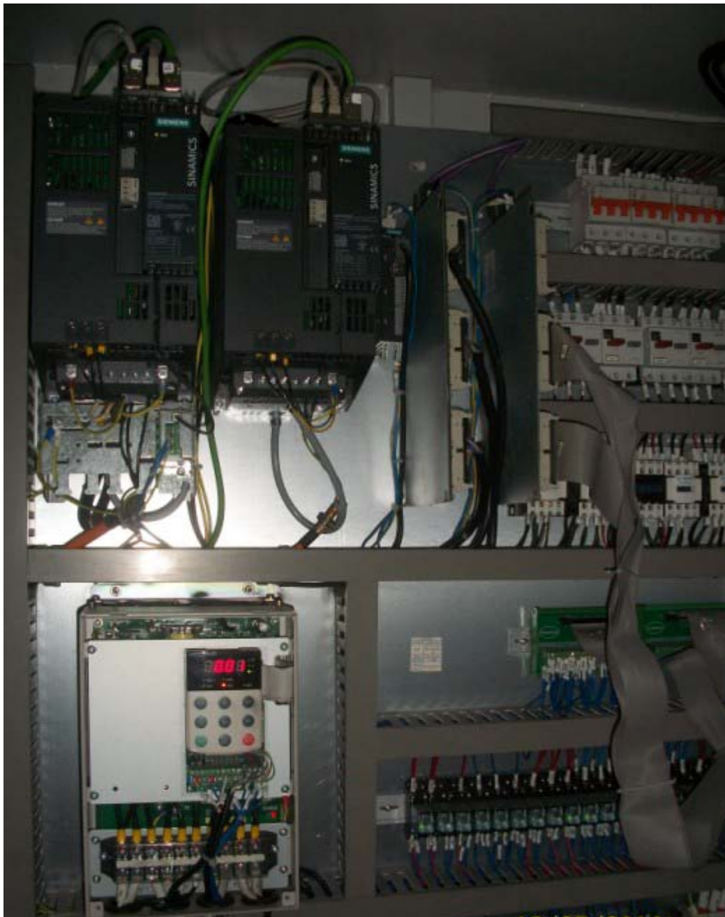
Figure 6 retrofits on machine tools with VSD drives on site
